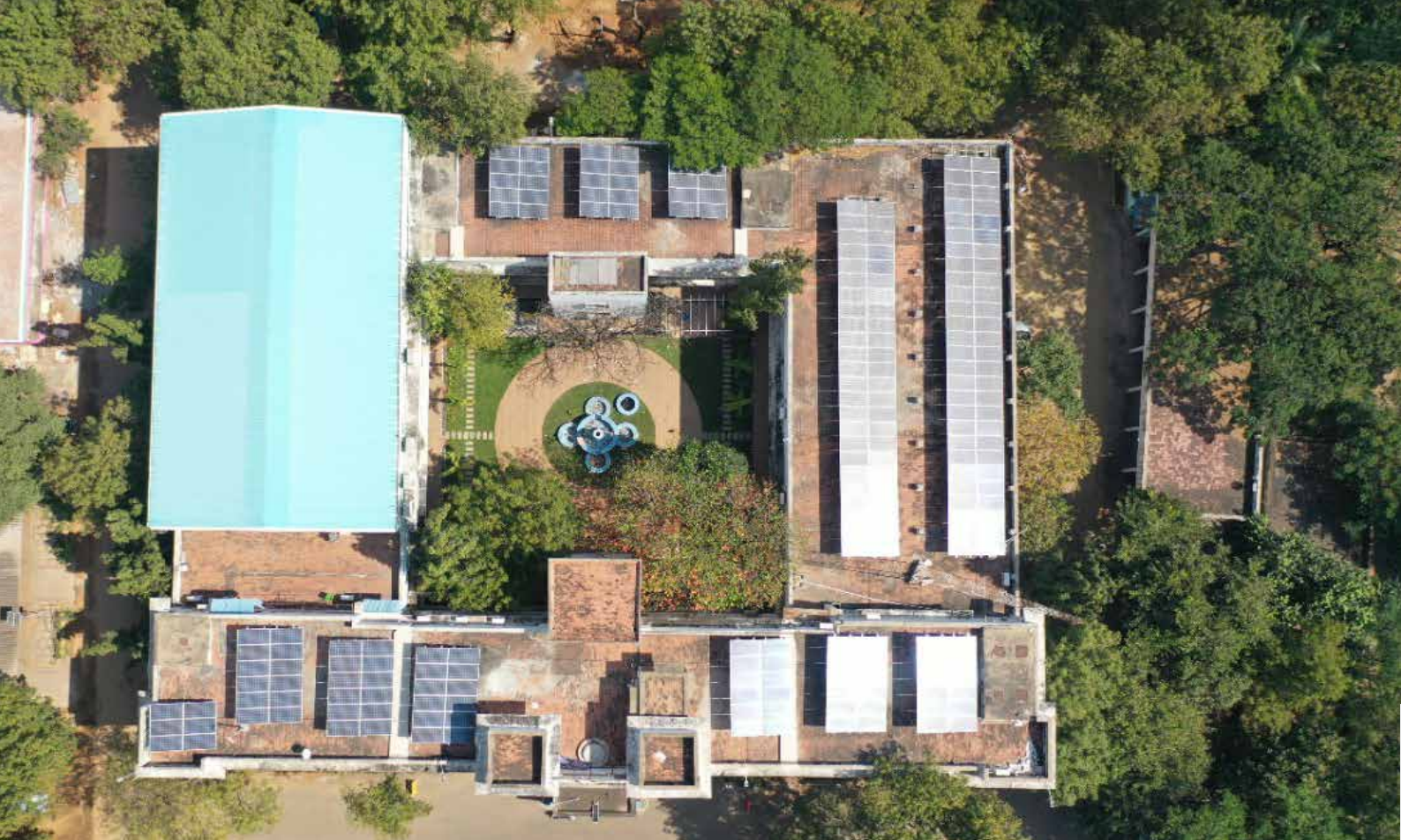
Figure 5: Solar Rooftop in Trichy Municipal Corporation Main Office
