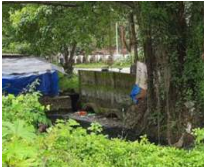
Figure 4-9: Blockage due to accumulation of solid waste
