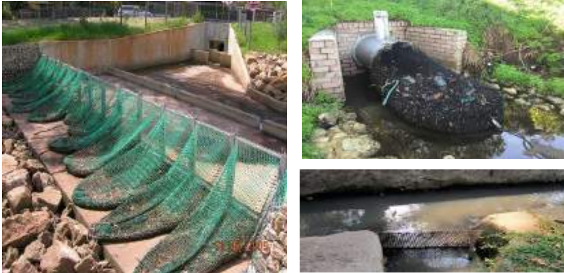
Figure 17: Trash Screens (Photo Credit: bechtel.org)
