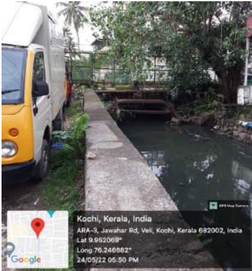
KWA Water pipeline aligned across the canal. At high flood levels in the canal the water pipeline can come in direct contact with the polluted canal water (Photo Credit: bechtel.org)
