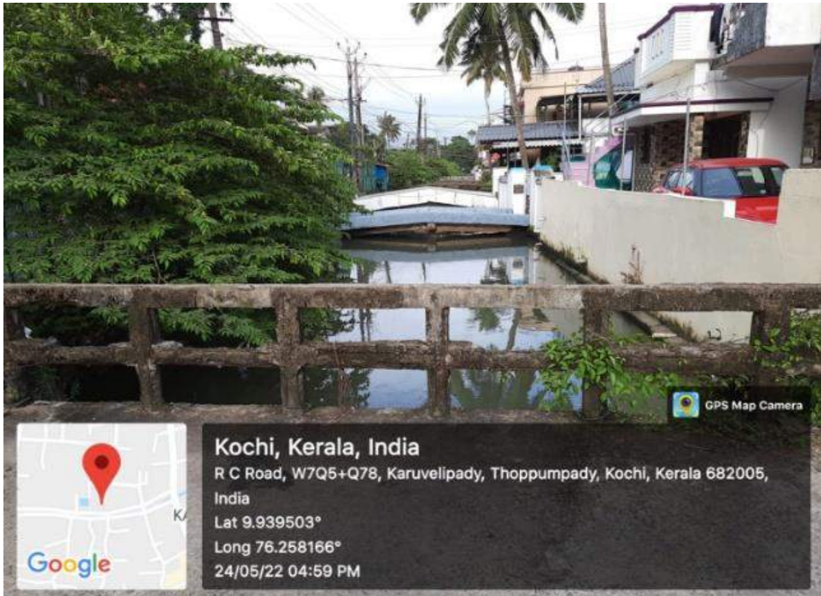
Footbridges built by each individual houses across the canal without ample headroom impedes the flow and cleaning operations (Photo Credit: bechtel.org)
