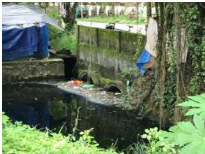
Figure 9. The bridge at Kochupally Road and the two culverts under the bridge.
