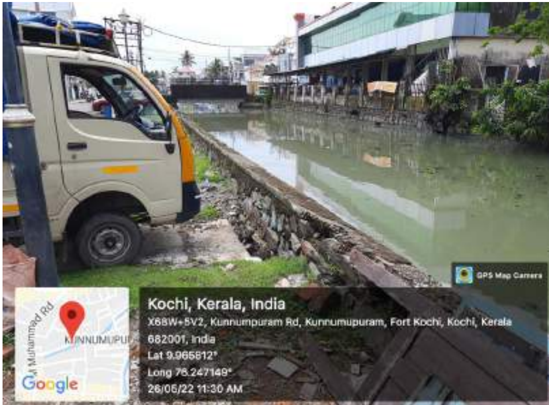
Canal Lining to be repaired (Photo Credit: bechtel.org)
