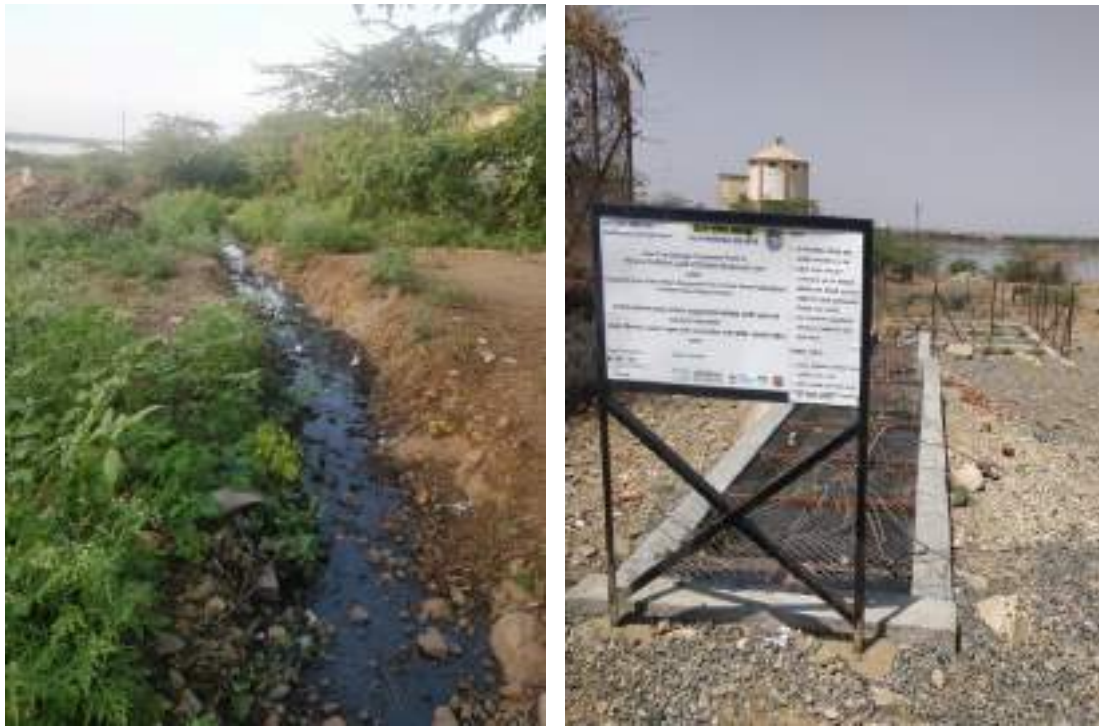
Figure 21: Constructed Wetland developed by ICLEI South Asia (Photo Credit: ICLEI South Asia)
