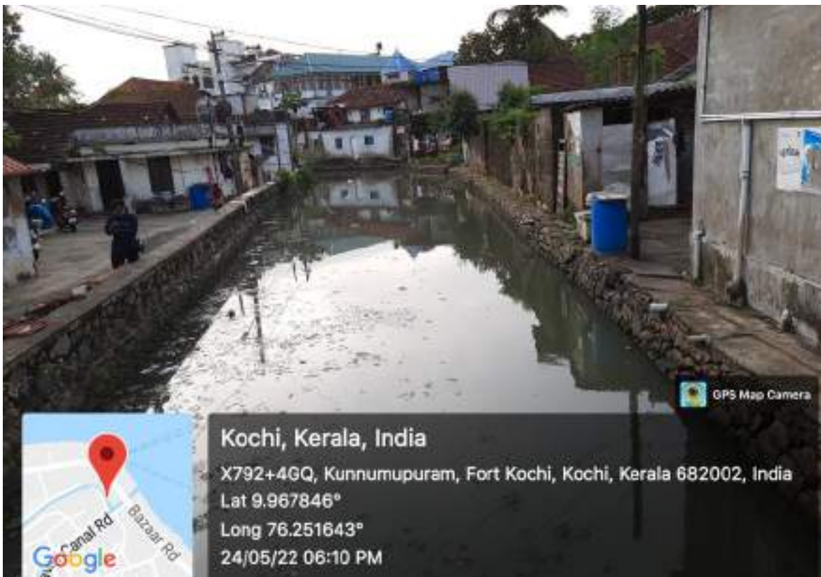
Grey and black wastewater getting discharged directly into the canal (Photo Credit: bechtel.org)
