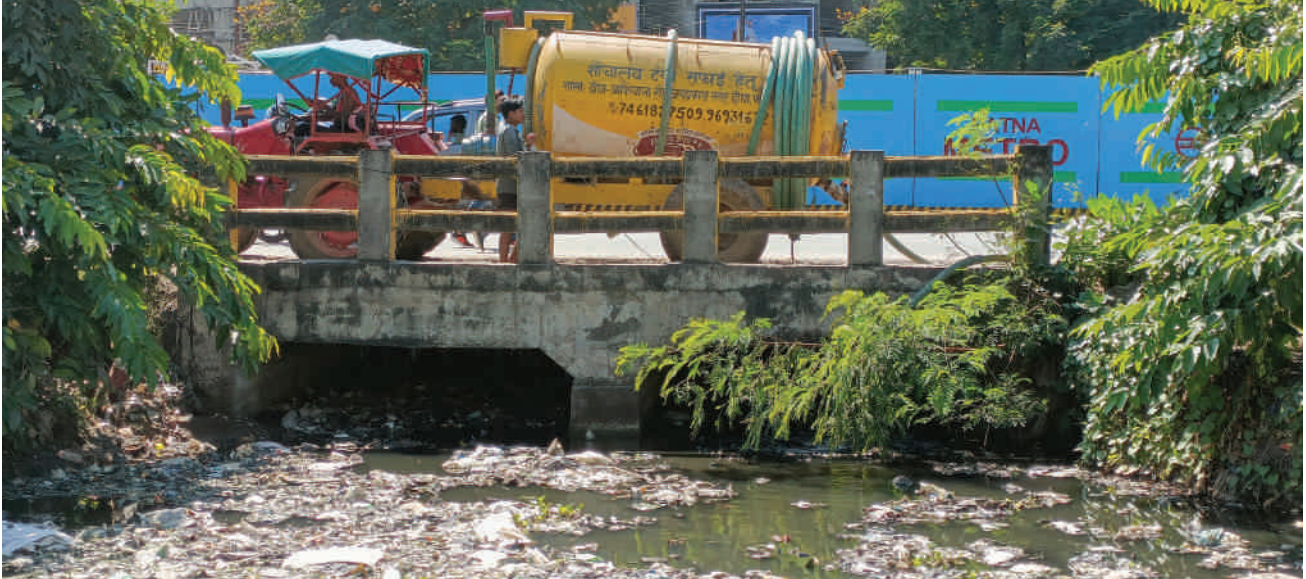
Open disposal of faecal sludge
