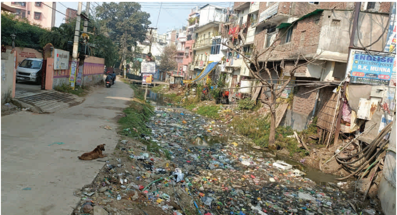
Stagnant Open Drain in Patna
