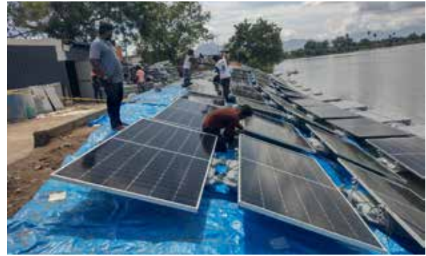
October 2024, Periyakulam Lake, Coimbatore, Tamil Nadu, India: The Coimbatore City Corporation issued a work order to ICLEI South Asia for the implementation of a 140-kWp Floating Solar PV plant at the lake, under the state's Namakku Naame scheme. The capacity of the pilot was then increased to 154 kWp to ensure policy compliance.
