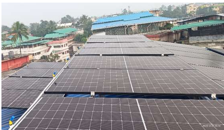
25 kWp Rooftop Solar PV System Installed at Siliguri Municipal Corporation Office
