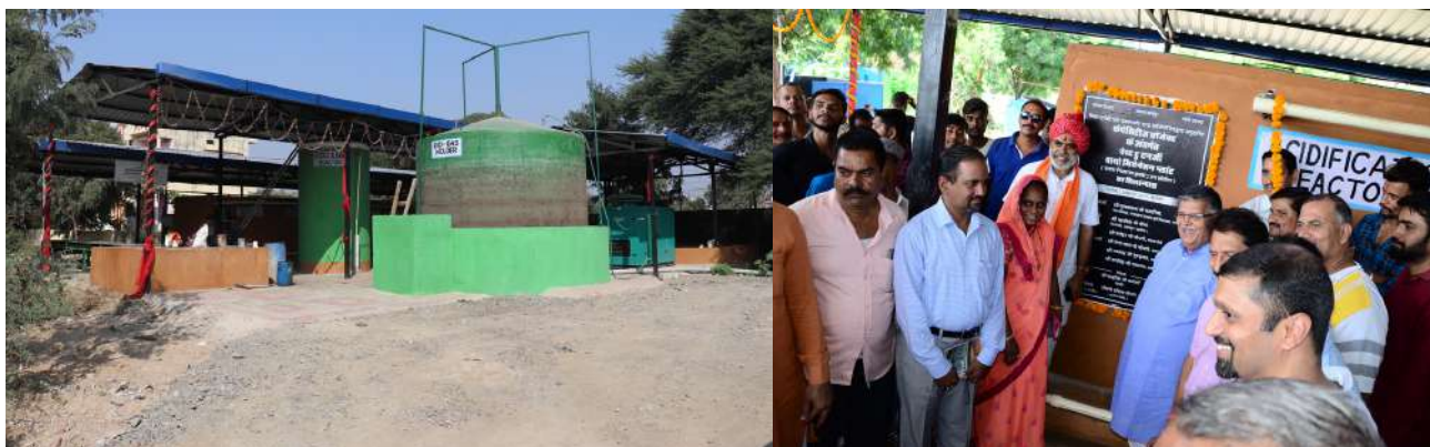
2 TPD Biomethanation Plant (Waste to Electricity) at Madri Fire Station and its Inauguration (From Left)
