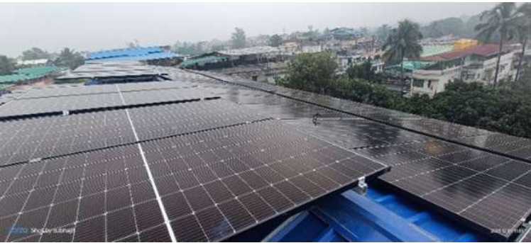
25 kWp Rooftop Solar PV System Installed at Siliguri Municipal Corporation Office
