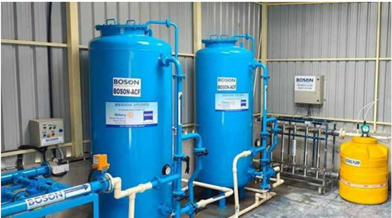
Figure 7: Tertiary treatment (Photo Credit: https://thebetterindia.com/373474/bengaluru-water-solutions-stp-treated-lake-rejuvenation-devanahalli-biome-environmental-trust-boson-whitewater/ )
